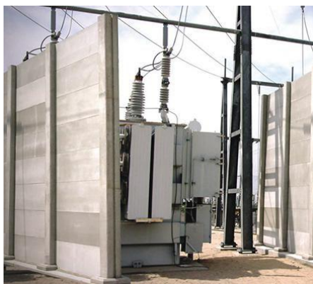
TruFireWalls protecting a substation transformer.
