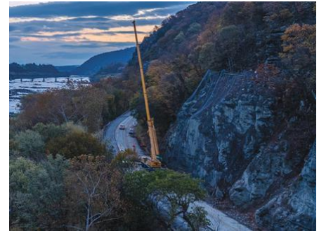
Rockfall hazards were mitigated along U.S. 340 in West Virginia by Access Limited Construction. Collaboration among departments of transportation was crucial because the project required a 22-mile detour affecting traffic in West Virginia, Virginia and Maryland.
