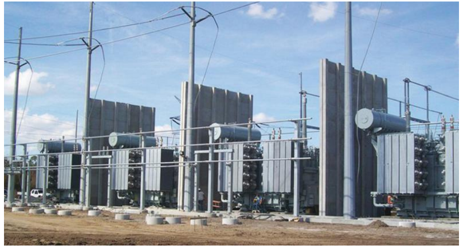
TruFireWalls installed at a substation.
