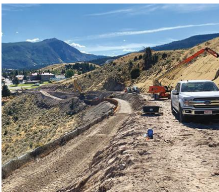
Access Limited and GeoStabilization International protect infrastructure from the unpredictable forces of nature, like at Yellowstone.
